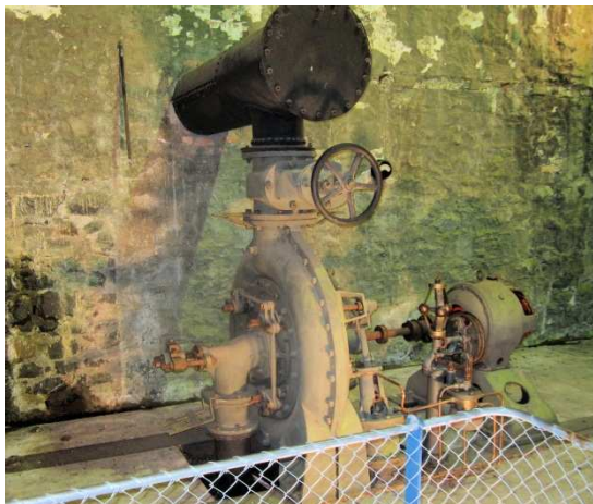
Duck Reach Water Turbine 1895
