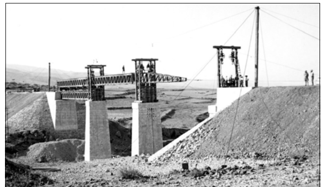
Nahr El Djadz - Image 5: The second and third spans, rigidly connected as one, are launched together, wheeled across the first span and hauled by a cable attached to the launching nose. Photo: ARHSnsw.
