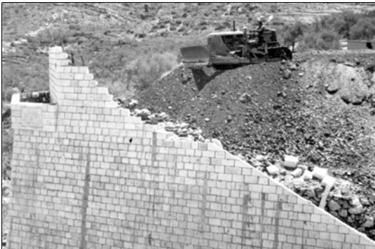
Nahr El Fgal - Image 3: The ARC&MG was well equipped - eventually. Here a bulldozer backfills behind the abutment. Photo: ARHSnsw.
