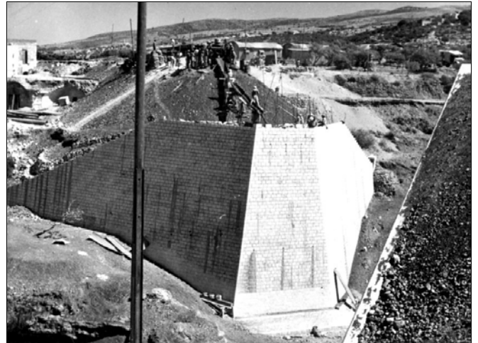
Nahr El Fgal - Image 2: The high abutment rises. Engineering design may have been Australian, but the wonderful masonry was Lebanese. One chute has been dismantled - the other is still operating. Photo: ARHSnsw
