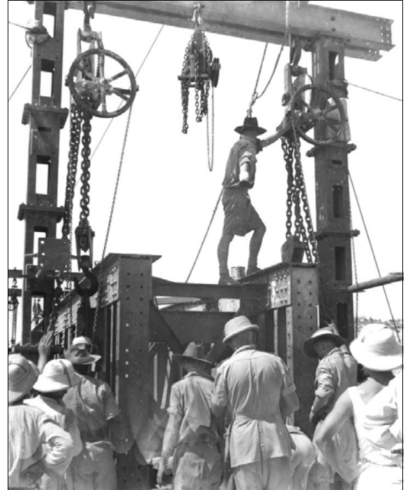
IMAGE at RIGHT: A group on an abutment watching a truss of a Nahr El Fidar Bridge span being lowered with chain blocks to its final position. Photo: ARHSnsw.
