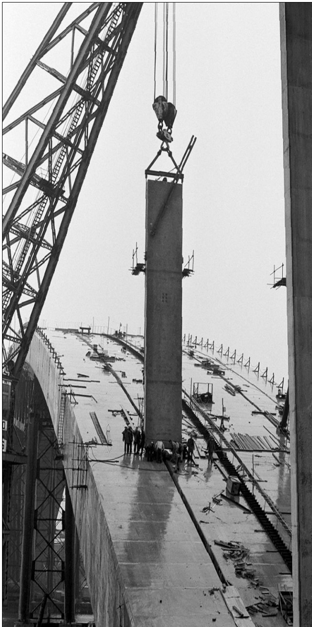
A precast concrete deck column lifted into place on the arch by the Titan crane. Photo: RTA neg16700 Aug 1963.
