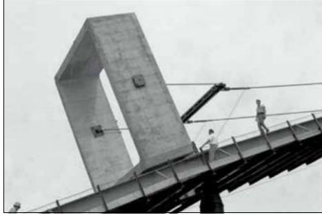
A box unit has been lifted to the crown of the falsework arch and is being slid down the arch to its seat. Photo: RMS January 1963.
