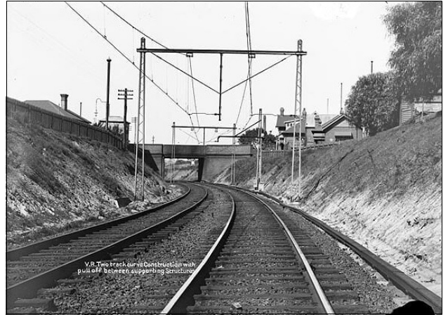
Victorian Railways two track curve construction on the Brighton line between Prahran and Windsor stations. Photo: April 1929, from PROV.
