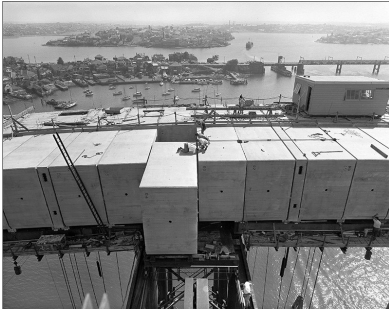
The last concrete box unit on the 2nd rib is slid into place. Note the narrow diaphragm units either side of the last box unit, also the original Gladesville Bridge in the background. Photo: RTA neg14526 taken 13 July 1962.
