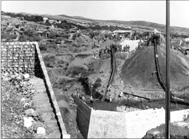
Nahr El Fgal - Image 1: The massive retaining walls of the high abutments. The stone facing acts as formwork for 2,000 tons of reinforced concrete behind. The abutment at left is almost completed. Across the ravine, two mixers feed wet concrete into chutes, filling up behind the masonry.. Photo: ARHSnsw.
