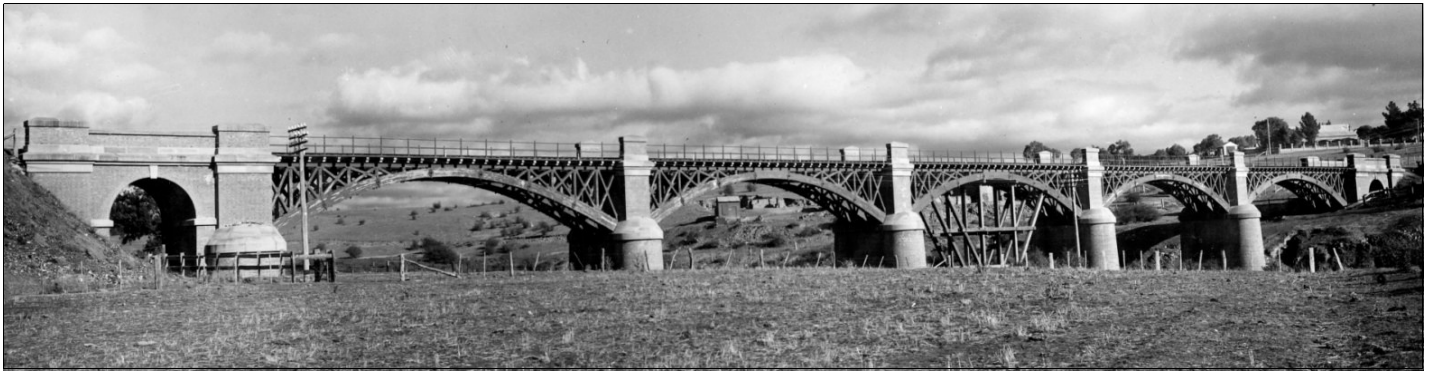
The timber arch bridge at Queanbeyan which was strengthened for the passage of the gun. The props under the centre arch may or may not be the work undertaken but they were erected about the same time. Photo No.1 008145b – Source Possibly NSW State Archives..
