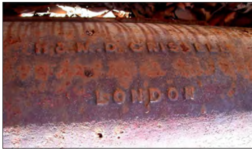
Detail of a branded column from the Grissell Building. Photo: courtesy GML Sydney.
