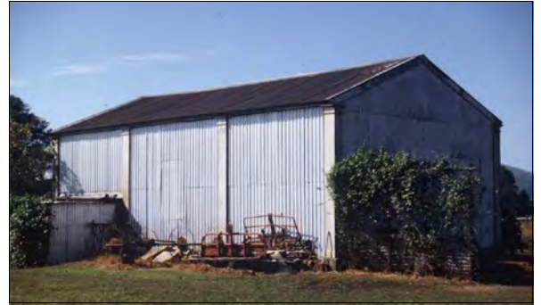
Former Presbyterian Church, Numbaa, New South Wales, 1855. Shows the face of the cast-iron stanchions along the wall. Photo: Miles Lewis.
