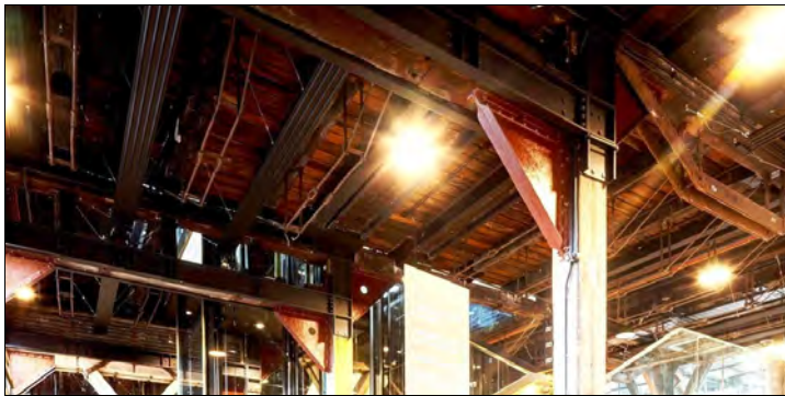
A lightened detail adapted from Brett Boardman's photo of the Foyer at the wharf level of Pier 2/3, showing the construction of the under floor level above.
