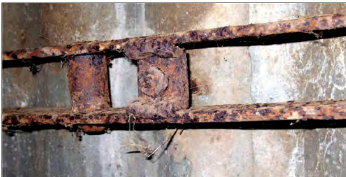
Interior detail of the iron shed at Longford House, Longford, Tasmania. Shows corrugated iron wall cladding bolted to an iron wall girt. Photo: Miles Lewis.
