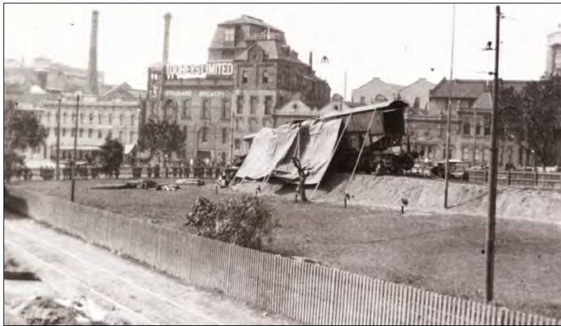
The obviously subsided gun ran through the end of its siding and derailed. Tarpaulins allow repair work to proceed and may be intended to exclude rain from the weakened embankment. April 1920.
